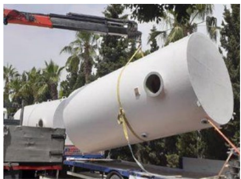
Recirculation tanks for brines and coagulants, July 2022
