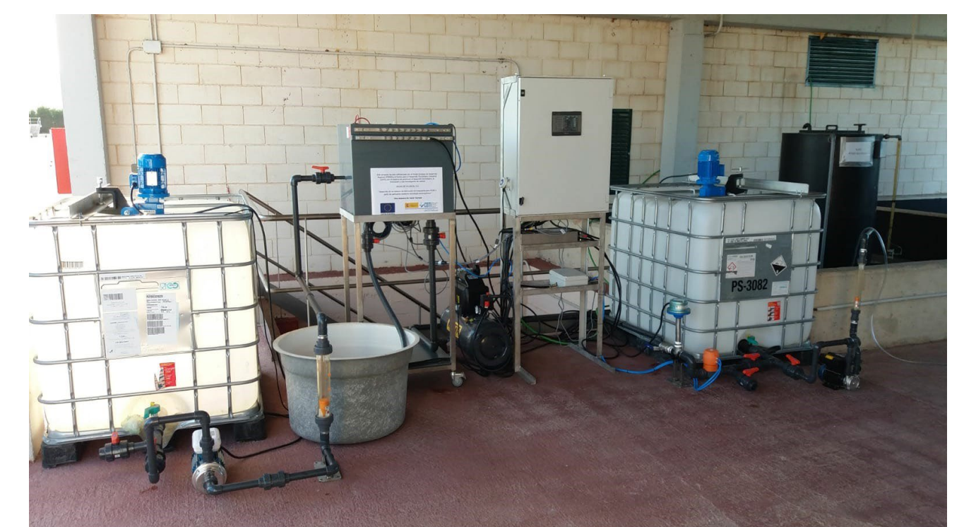
Figure 3- Pilot plant for coagulants production.
